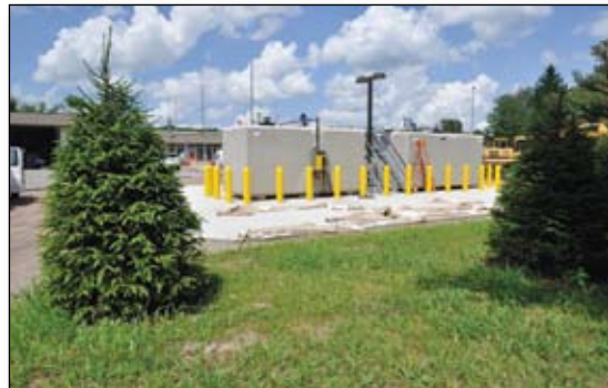
Final above ground storage tanks
